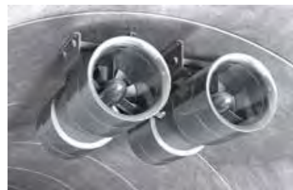
Ventilatori in tunnel
